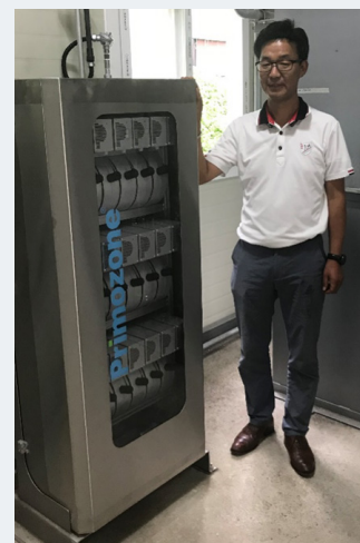
Project Manager, Mr T Park from PAOR next to the ozone system and in front of the re-circulation tank
